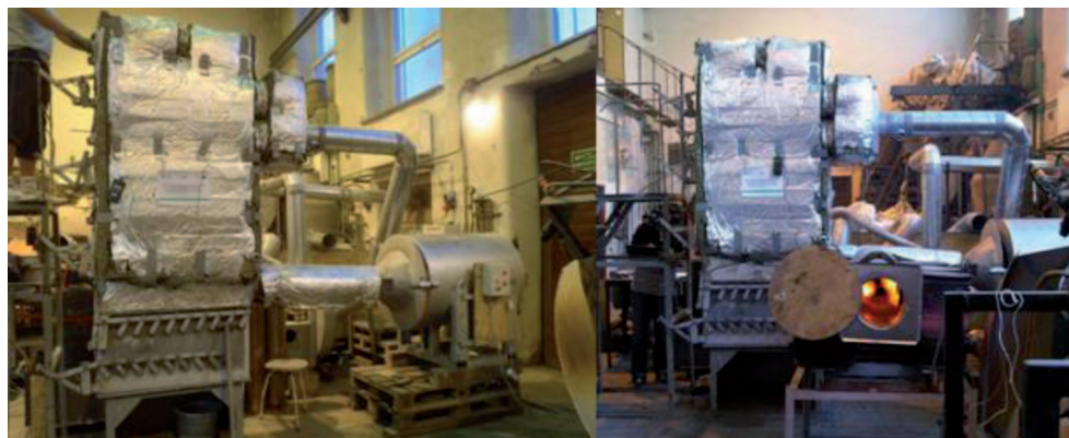
Fig. 6. View of the new dryer
