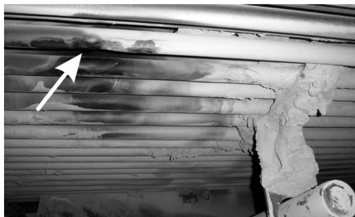
Fig. 1. Superheater failure caused by erosive action of ash carried away with the steam stream of soot blower's jet. Arrow indicates the location of steam leakage
