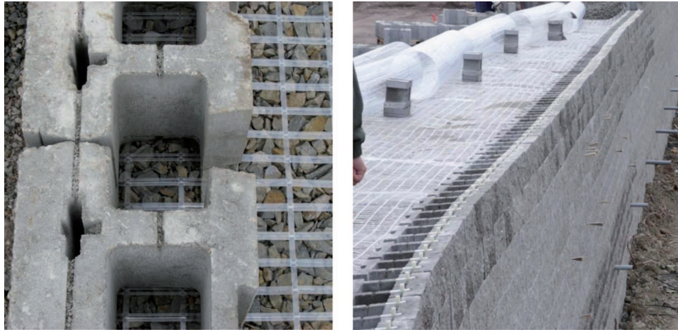
Fig. 12. Block wall with friction connection under construction, Zanovica (SK), 2009, (Vollmert et al., 2010).
