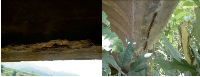
(a) Arch rib damage and rib exposure (b) Arch rib damage and rib exposure
