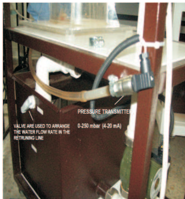
Fig. 4. Photo of pressure transmitter and valve
