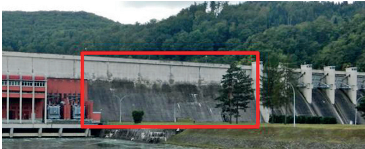
Fig. 6. View of the vented wall of the Rożnów water dam with the scanned area red-marked
